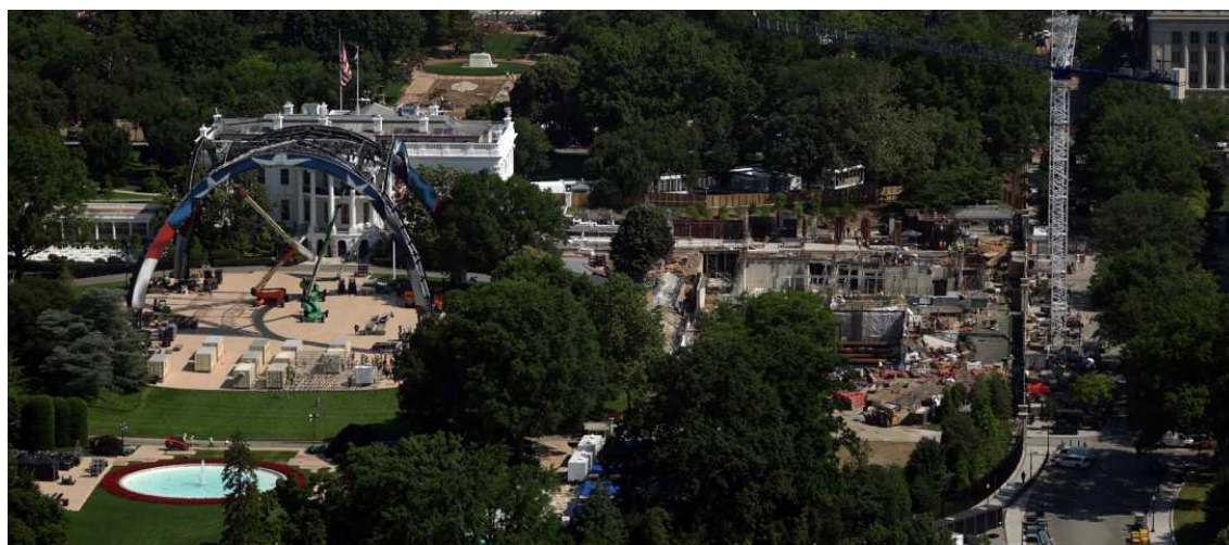
Construction continues for the upcoming UFC match alongside the ballroom addition on the South Lawn of the White House on May 28 in Washington. President Donald Trump is hosting a UFC match on the White House grounds to mark the 250th anniversary of the U.S. ALEX WONG/GETTY
