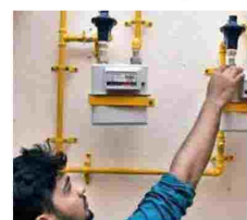
PIPED GAS. The way forward
