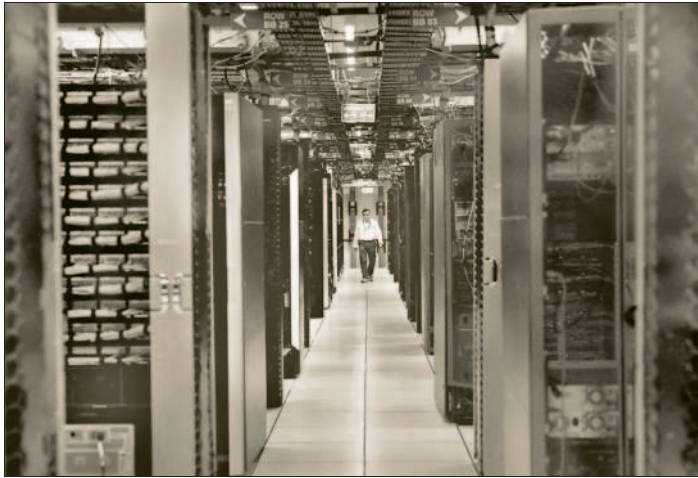
Each hyperscale data centre draws as much electricity as an aluminium smelter and consumes millions of gallons of water daily for cooling. REUTERS
