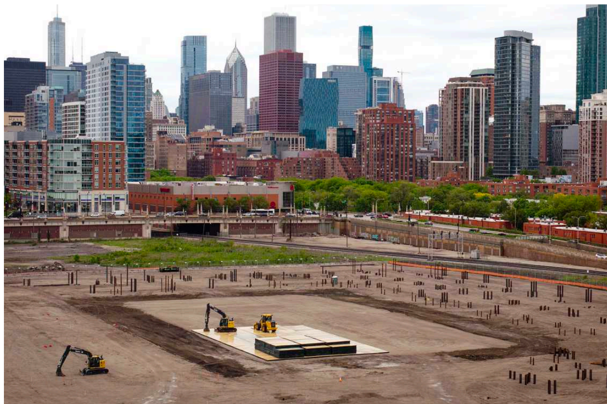
The 22,000-seat Chicago Fire soccer stadium is under construction at the north end of The 78 development in Chicago's South Loop on Tuesday. McDonald's has acquired naming rights for the new stadium, and it will be called McDonald's Park. E. JASON WAMBSGANS/CHICAGO TRIBUNE
