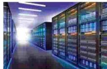
DATA CENTRES. Cooling implications
