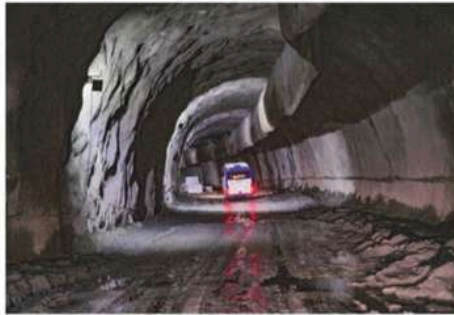
14 km-long under-construction tunnel at Zojila which will connect Sonmarg in the Kashmir valley to Drass in Ladakh — will allow the transportation of troops and supply by road all year round. This will make it easier to mobilise forces in times of need, and also cut costs associated with air transportation. Currently, the Army relies on transport aircraft from the Air Force for maintaining its
