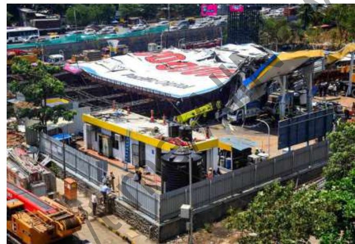
Deadly fall: Rescue and relief work underway at the site of the hoarding collapse at Ghatkopar, in Mumbai, on May 14. PTI
